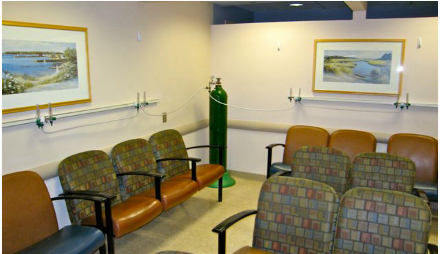
Figure 2-13: Portable, High-Capacity Gas Delivery Combined with an Equipment Rail Outlet System
