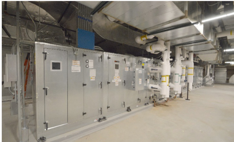
Figure A4-3: Genesis Health System's Air-Handling Units
